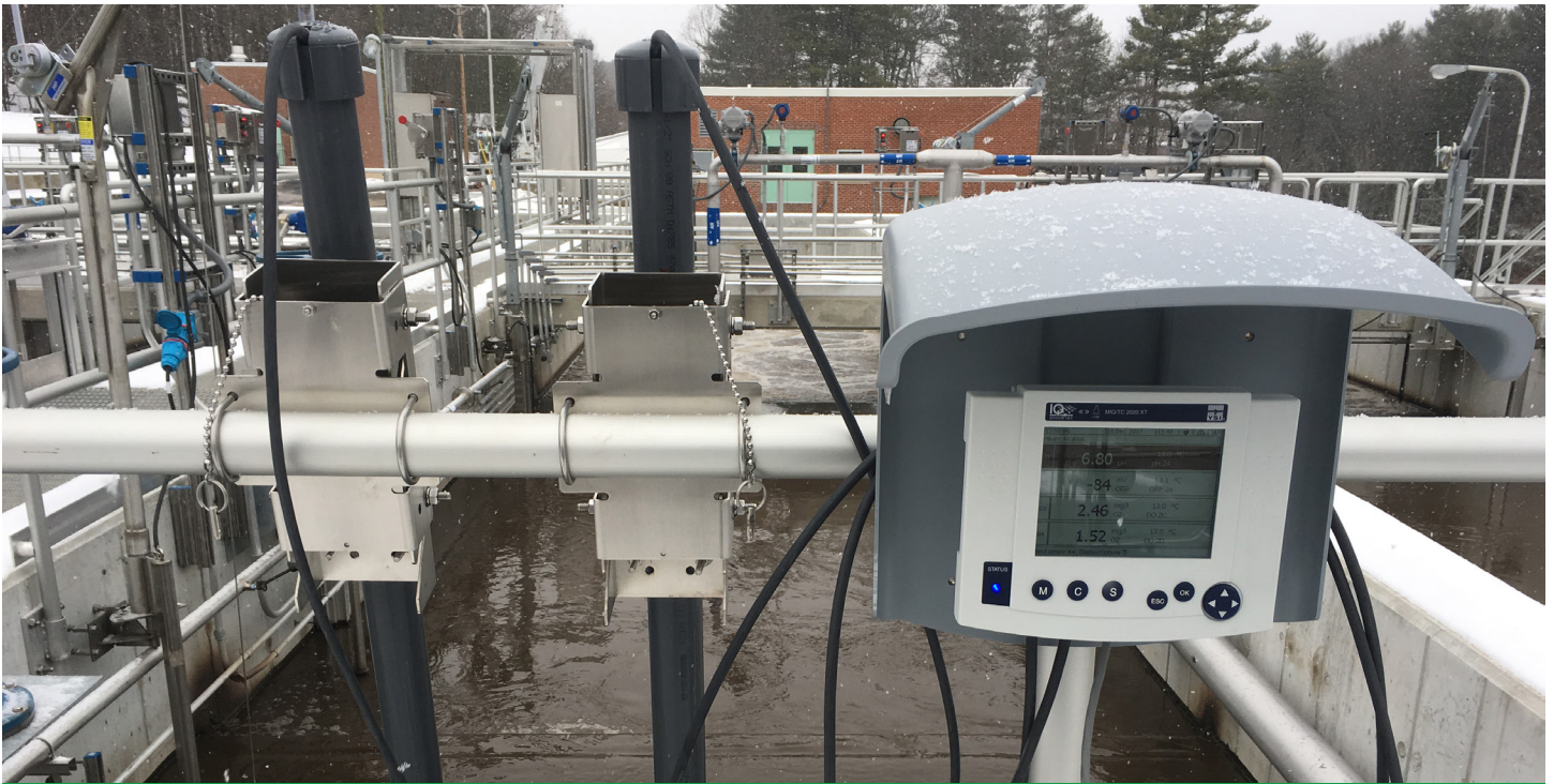
IQ SensorNet utilizes one controller to monitor up to 20 parameters on a single network. Newmarket decided to use two IQ controllers (one on each train) to monitor all 18 sensors in their activated sludge process.
